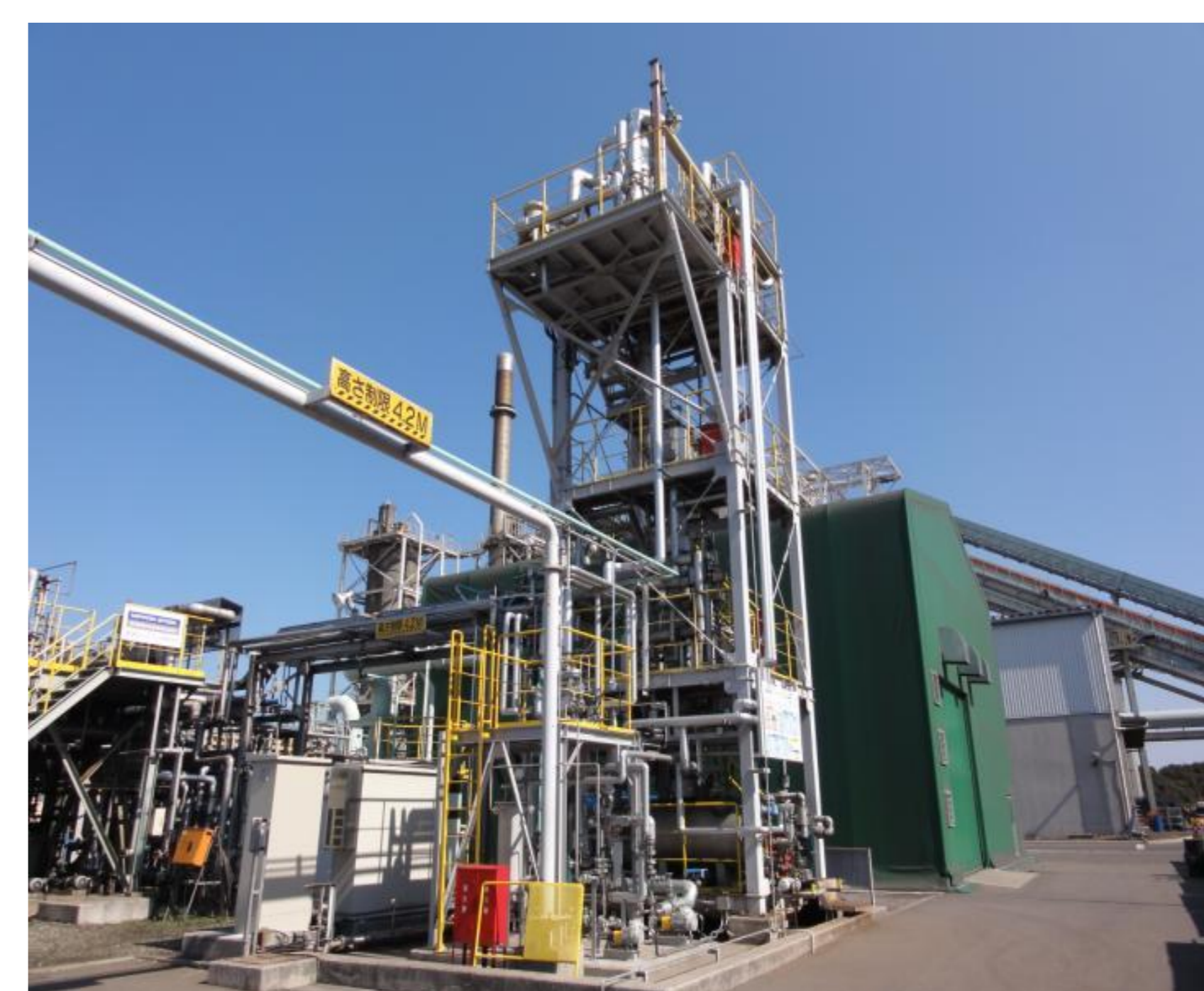
Pilot self-heat recuperative distillation for bioethanol Nippon Steel Engineering Kitakyushu Environmental Technology Center
